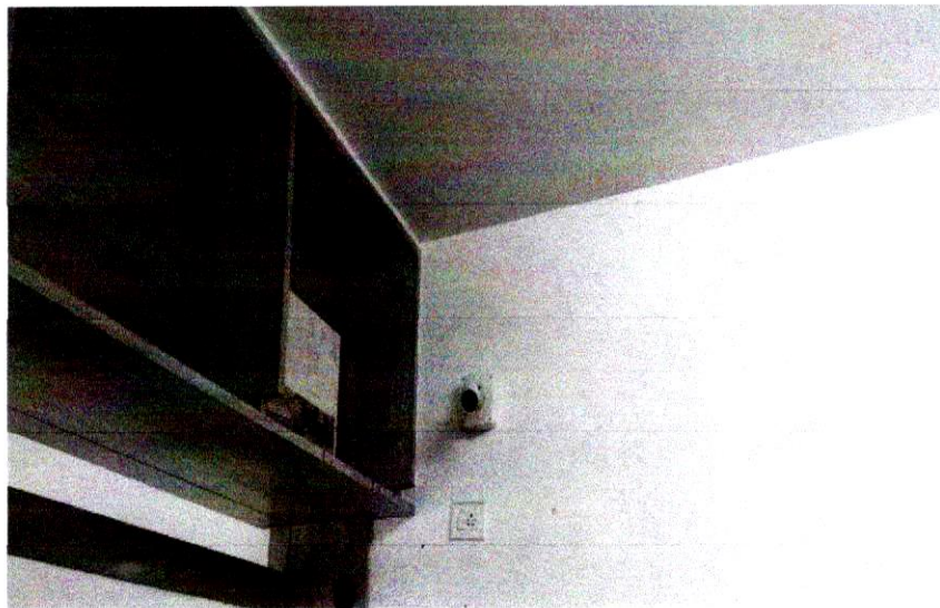
CCTV in Staff Room
