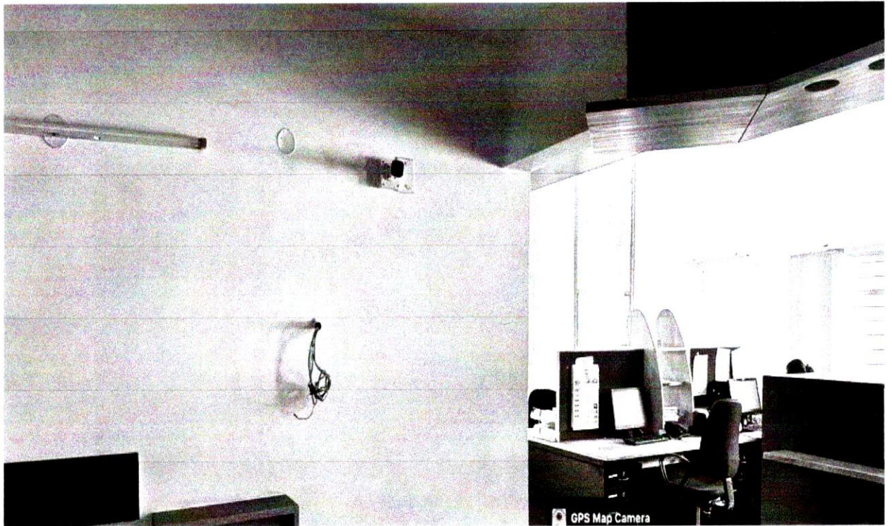
CCTV in Office Room
