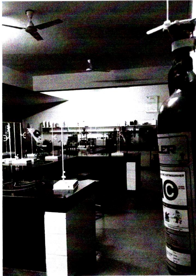
Fire Extinguisher in Laboratory
