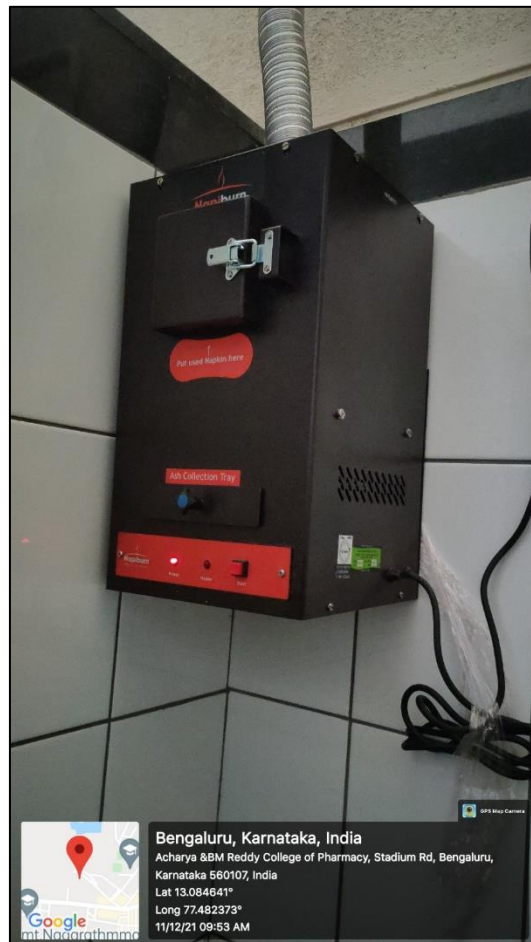
Sanitary Napkin Incinerator Installation at Women's Rest Rooms
