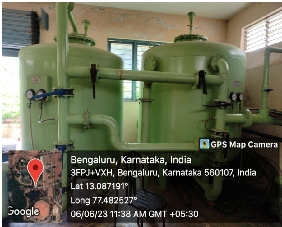
STP Plant Tanks
