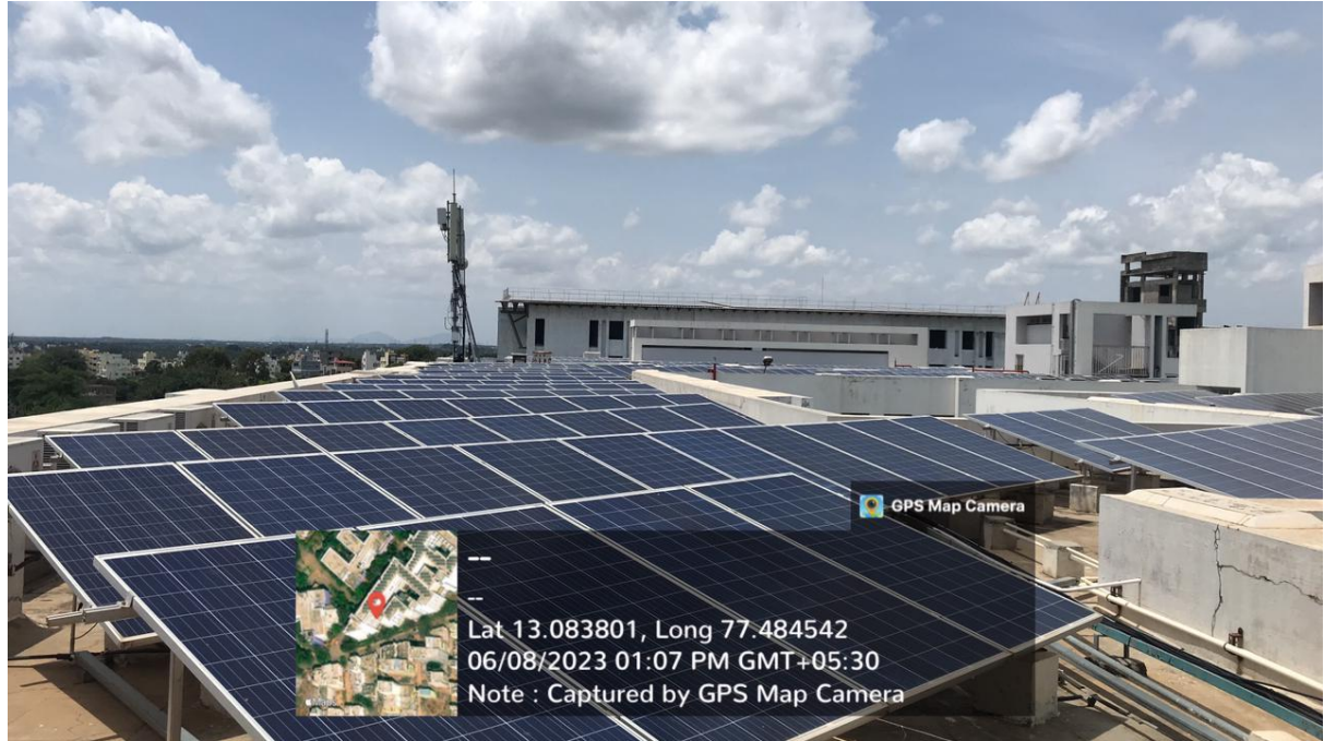
Photos of Solar Panels
